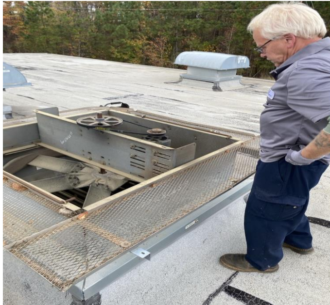
*Pictured above; Maintenance Tech Will Spani installs new belt on exhaust fan.
