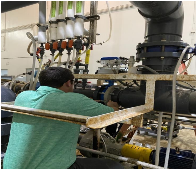
*Pictured above; Brice Doolittle is tightening bolts on new 6-inch CIP valve.
